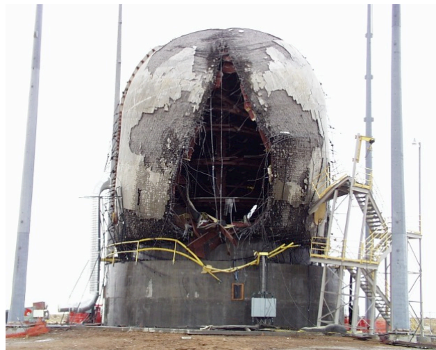
Figure 8 : Containments will not crack and reclose; they will burst. Results of SANDIA joint Japanese-U.S tests.
